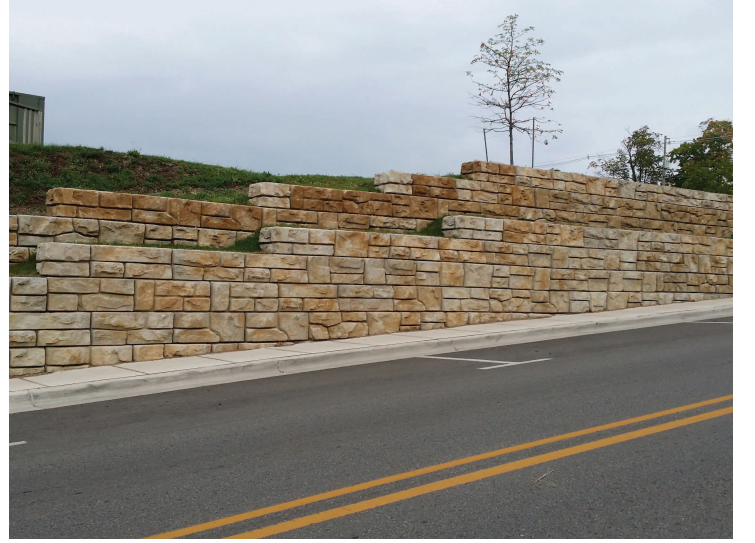
The retaining wall on State Street made from a concrete product produced in Charlevoix.
